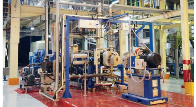
New polypropylene pelletizing line in Indonesia, with Useon's SAT-X 175 co-rotating twin-screw extruder; skid-mounted BKG® underwater pelletizer is in foreground
